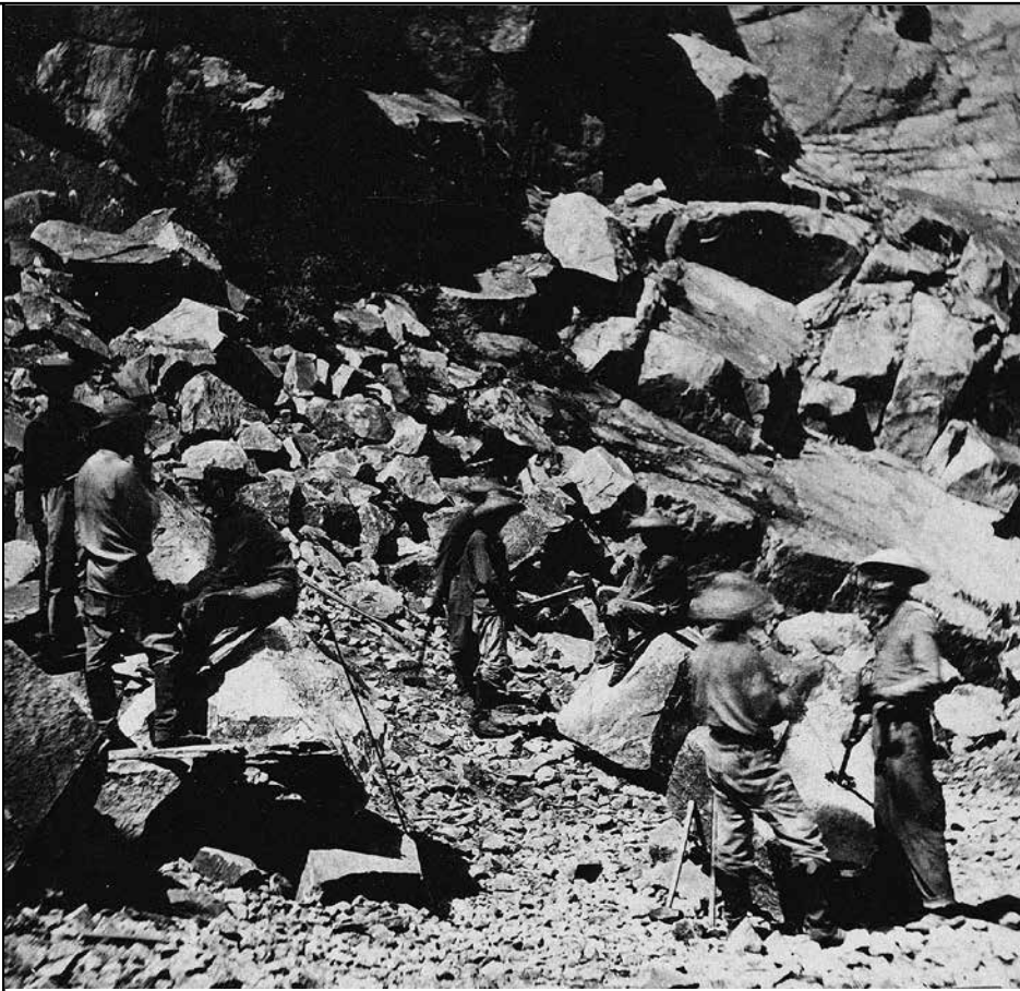
Chinese railroad workers breaking up rock. Note the sledge hammers and drill bits.
